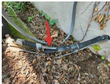
Right side - refrigerant line insulation.
