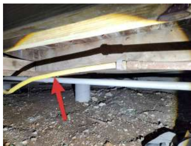
Crawlspace - CSST gas line.
