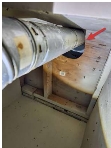
Furnace exhaust vent.
