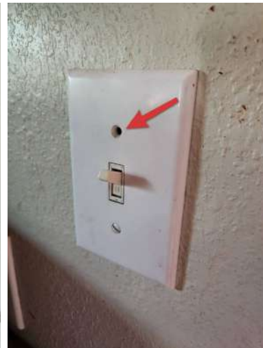
Kitchen switch - missing screw.
