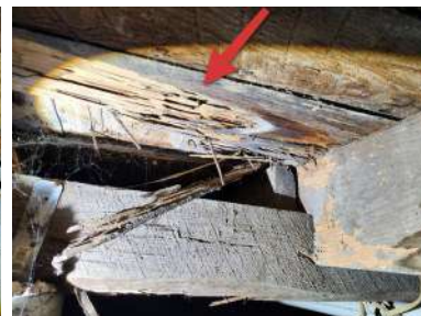
Subfloor - termite damage.
