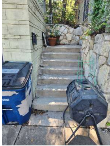
Front stairway - missing handrail.
