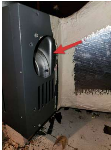
Furnace box - missing cover.
