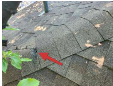
Back hip - damaged shingle.
