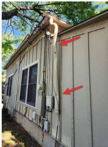
Right side - damaged downspout.
