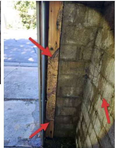
Left side - excessive moisture and organic growth.
