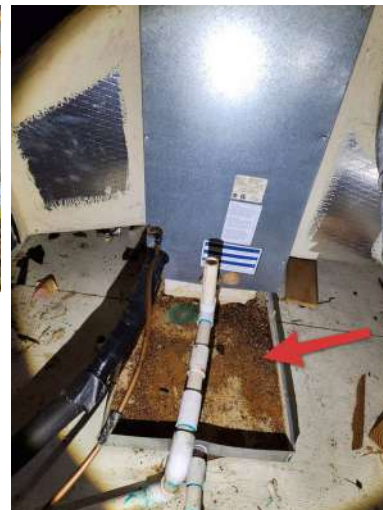
Attic, emergency pan - rust.
