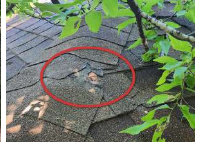
Back hip - damaged shingle.
