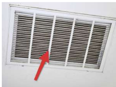
Hallway - air filter.
