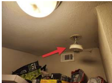
Laundry room - smoke detector.
