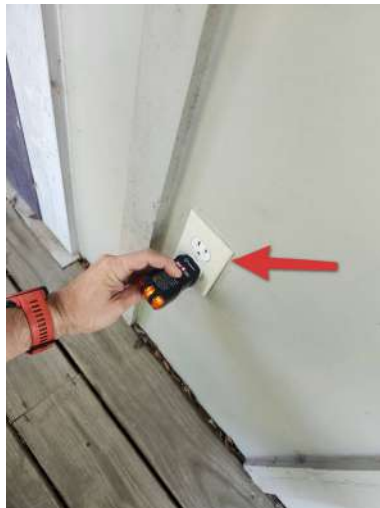
Front - not GFCI protected.
