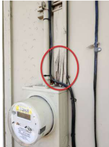
Right side - damaged trim board.
