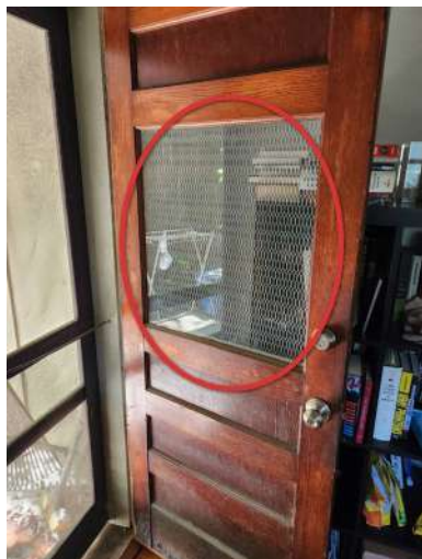
Back door - missing marked safety glass.
