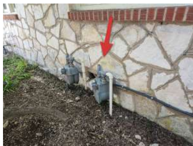
Left side - gas meter.
