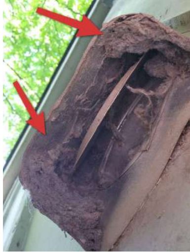
Back - dryer exhaust vent.
