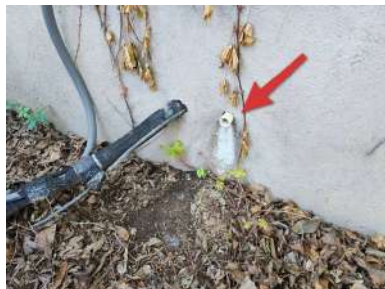
Right side - A/C condensation drain line.
