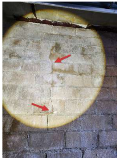
Right side - crack.
