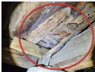
Subfloor - termite damage.
