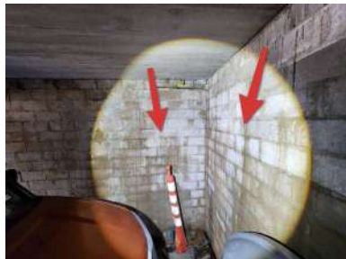
Back - excessive moisture.
