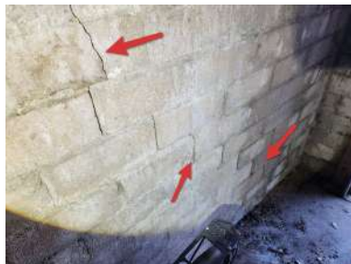
Right side - crack.
