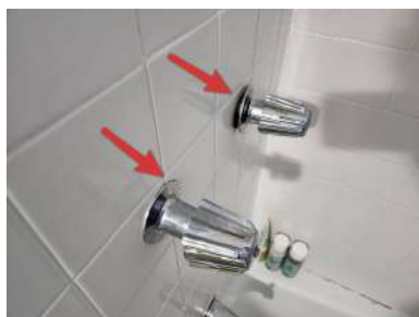
Bathroom - water valves.
