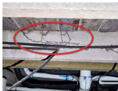
Beam - mud tubes (termites).
