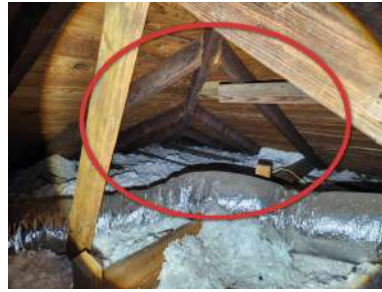
Missing brazing and vertical support.
