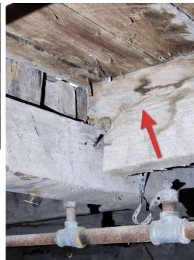
Beam - previous water leaks.
