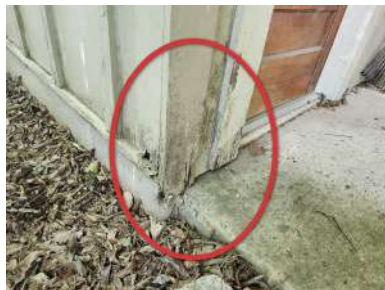
Back - damaged corner trim.
