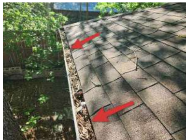
Left side - dirty gutter.
