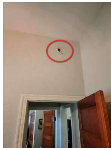
Bedroom - missing smoke detector.
