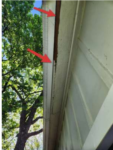
Left side - damaged soffit.
