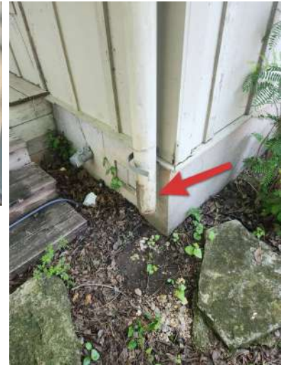
Front-right - damaged downspout.
