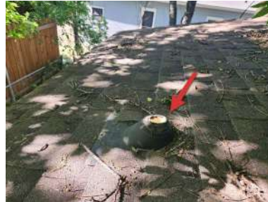
Back - short plumbing vent.
