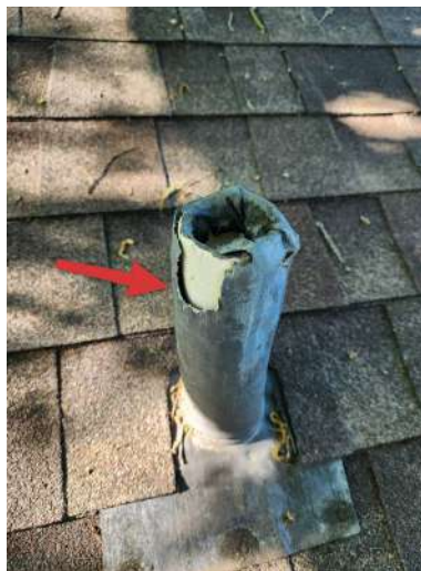
Left side - damaged plumbing vent.
