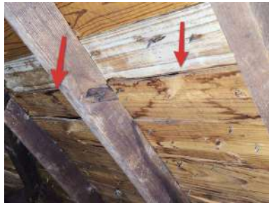
Previous water leaks.
