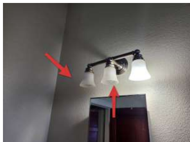
Bathroom - inoperable light bulbs.
