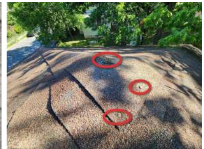
Ridge - exposed fasteners.
