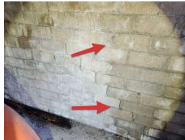
Right side - excessive moisture.
