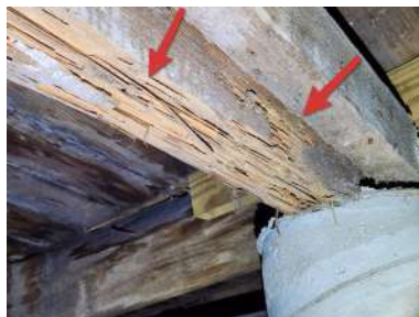
Beam - termite damage.
