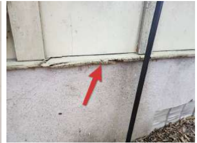
Right side - damaged siding.
