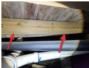
Beam - previous repairs.
