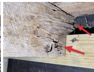
Beam - termite damage.
