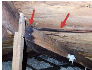
Previous water leaks.
