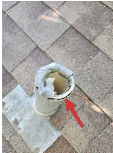
Right side - damaged plumbing vent.
