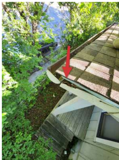
Front-right - damaged fascia.
