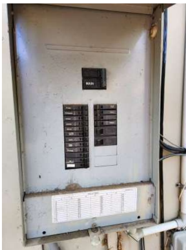
Right side - main electrical panel.
