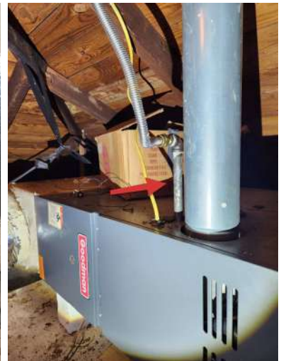
Gas supply line - missing sediment trap.
