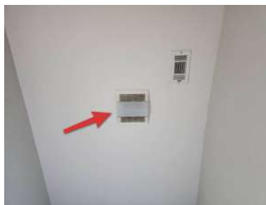
Bathroom exhaust vent.
