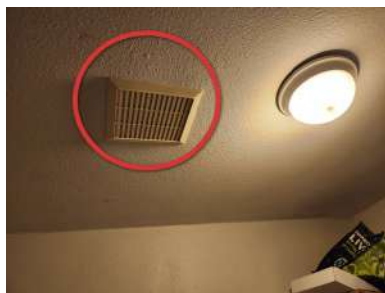
Laundry room - inoperable exhaust vent.
