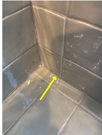
GAPS / CRACKS AT TUB
