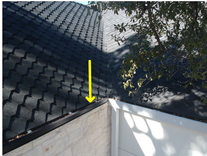
DEBRIS IN GUTTERS -view of recessed gutter
