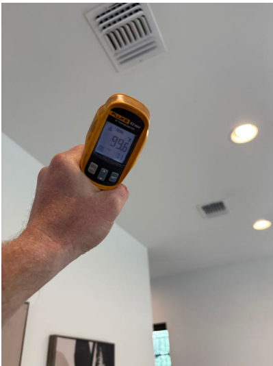
DOWNSTAIRS FURNACE ZONE WAS FUNCTIONAL
