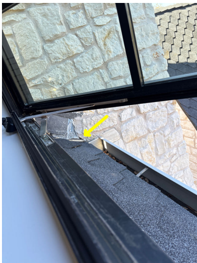
MISSING KICK-OUT FLASHING -above chimney
