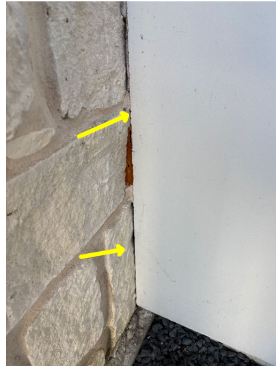
GAPS BETWEEN SIDING
