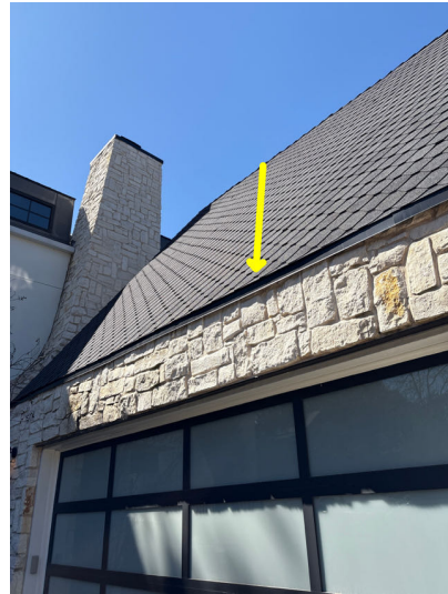
No gutter / no eave
