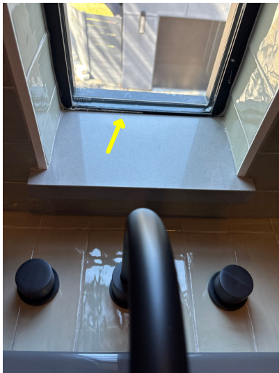
GAPS / CRACKS AT TUB
