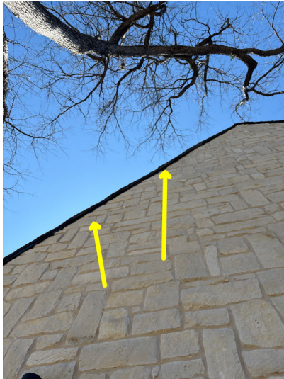
Gaps behind garage drip edge -weathered roof decking visible
