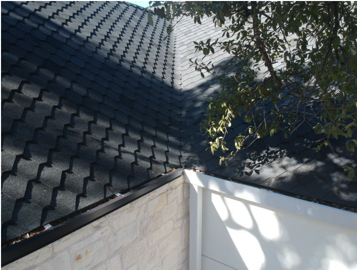
TREE IN CONTACT WITH SHINGLES
