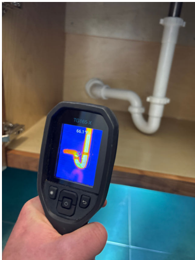
NORMAL THERMAL READINGS - DRAINS
