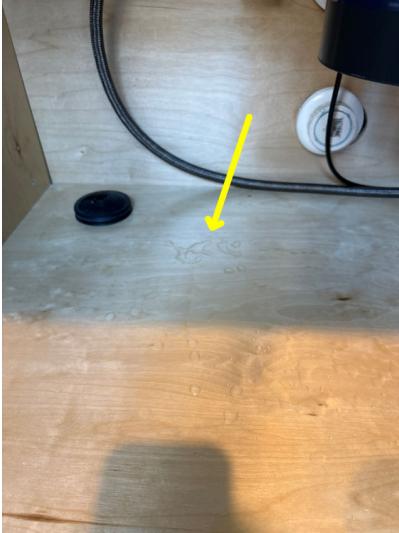
Water in cabinet below kitchen sink
