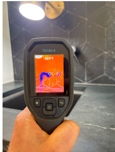
NORMAL THERMAL READINGS - WATER LINES
