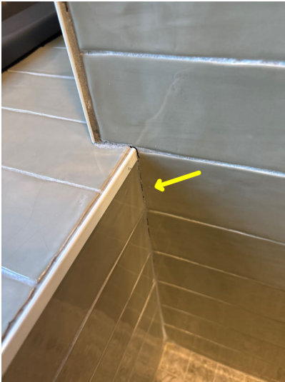
GAPS / CRACKS AT SHOWER
