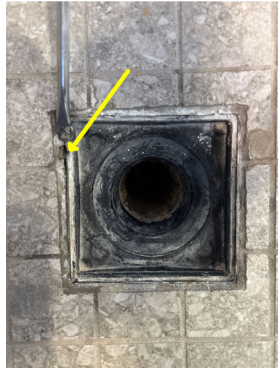
GAPS / CRACKS AT SHOWER
