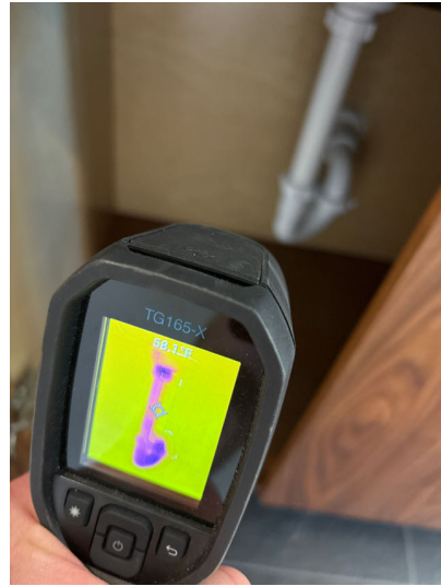
NORMAL THERMAL READINGS - DRAINS
