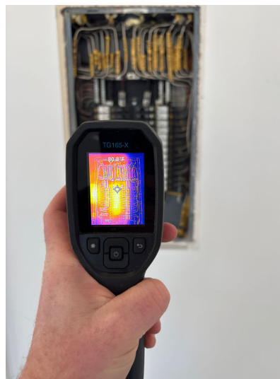
NORMAL THERMAL READINGS - SUB PANEL
