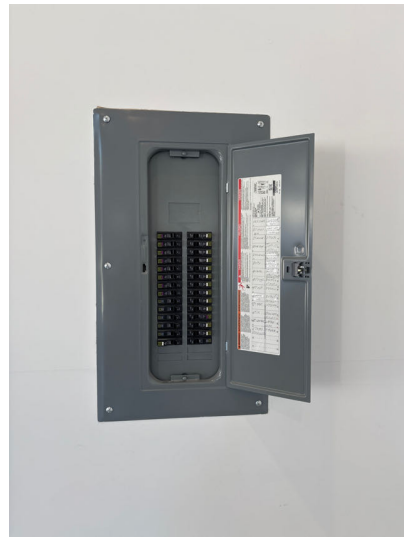
NO MAJOR ISSUES - SUB PANEL
