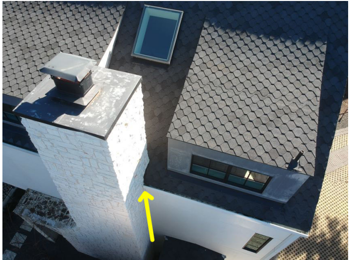
MISSING KICK-OUT FLASHING
