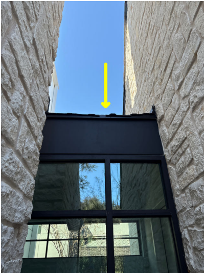
No gutter / no eave
