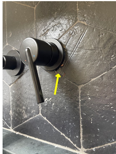
Damaged tile -bar area
