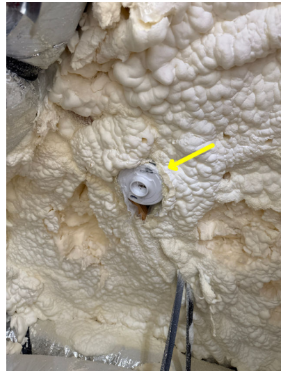
ATTIC LIGHT BULB IS MISSING
