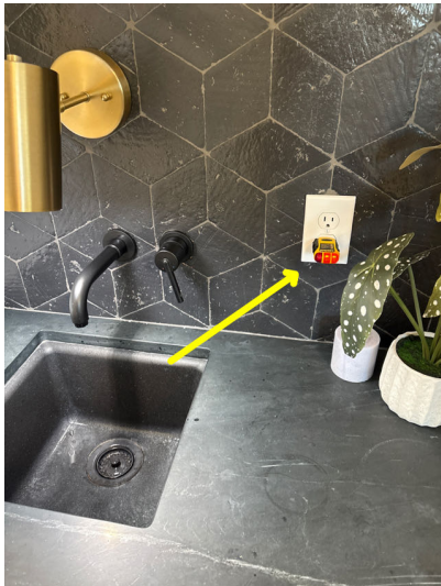
GFCI PROTECTION MISSING -bar
