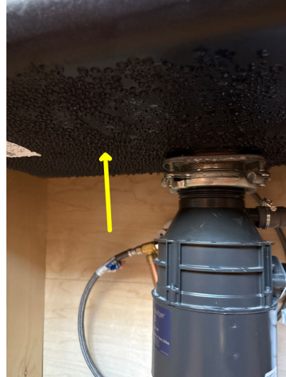
Water beading below sink basin
