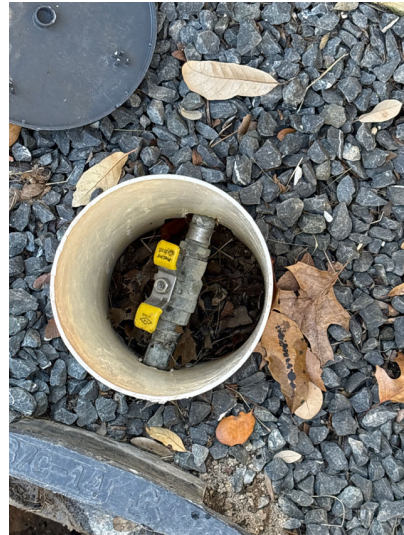
Water shut off
