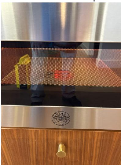
NO MAJOR ISSUES - MICROWAVE
