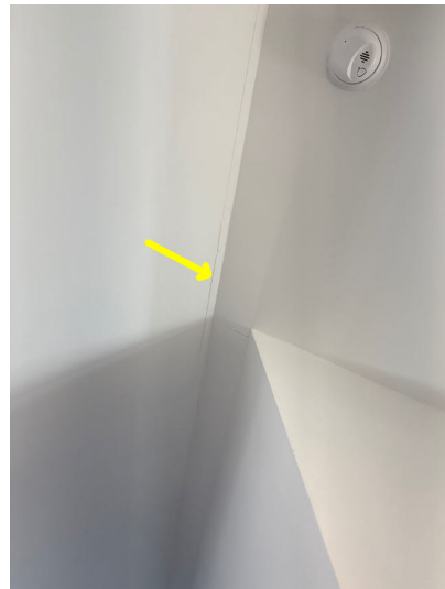
INTERIOR SETTLEMENT CRACKS
