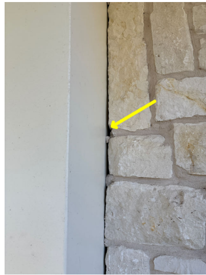
GAPS BETWEEN SIDING
