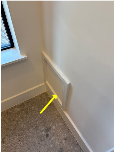
Tub access panel is painted to the wall. Not removed for inspection
