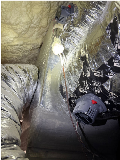
PROPERLY SEALED DUCTS
