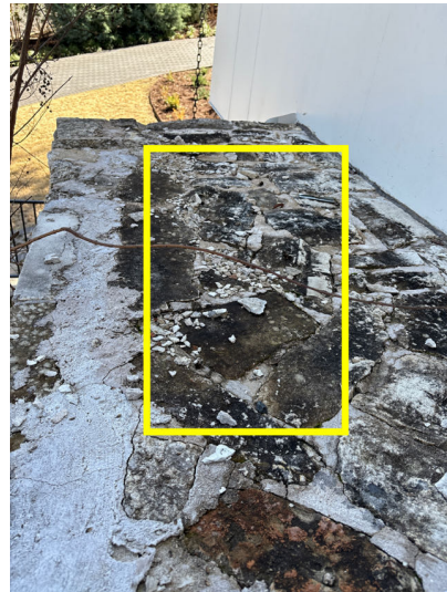
LOOSE MORTAR JOINTS -entry arch
