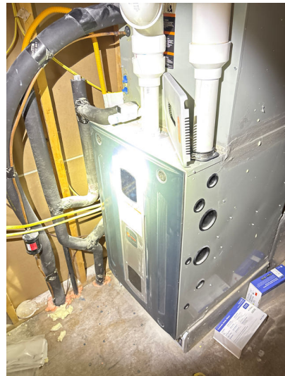
PROFESSIONAL INSTALL - FURNACE
