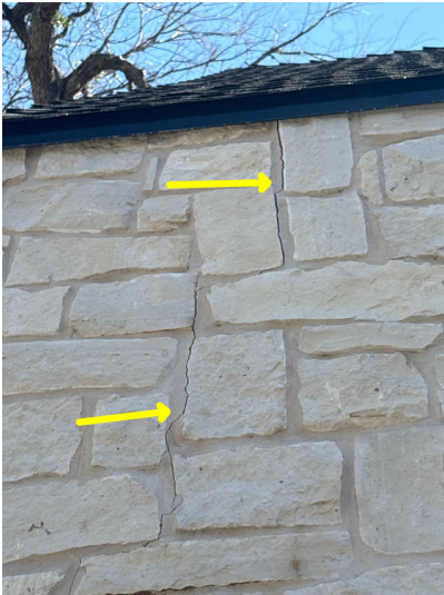
EXTERIOR SETTLEMENT CRACKS
