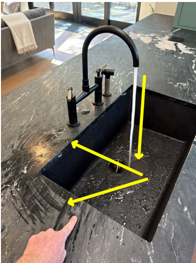
Water running in the sink splashed out more than what is considered normal
