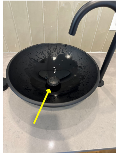
DRAIN STOP NOT FULLY FUNCTIONAL
