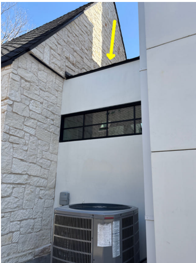
No gutter above HVAC condenser
