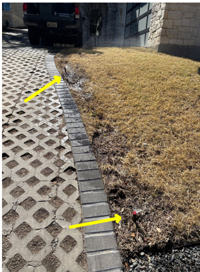
Sprinklers run over with vehicles are functional
