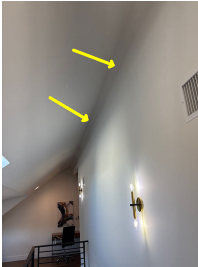
INTERIOR SETTLEMENT CRACKS
