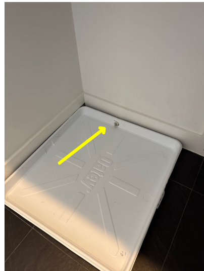
Disconnected washing machine drain
