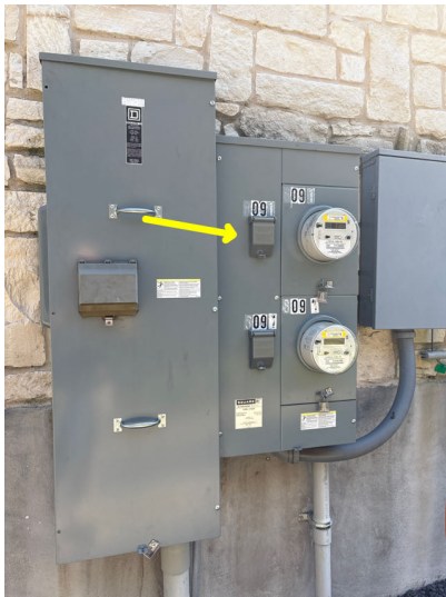
MAIN BREAKER FOR UNIT 1
