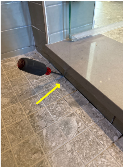
GAPS / CRACKS AT SHOWER
