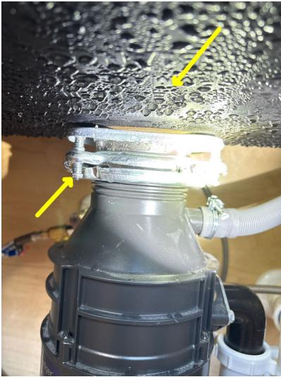
Water dripping from disposal flange
