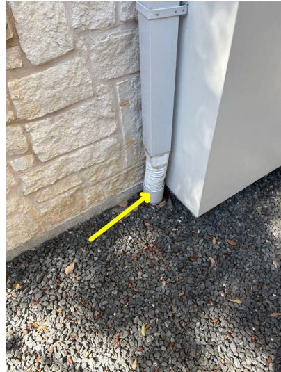
Below grade drains
