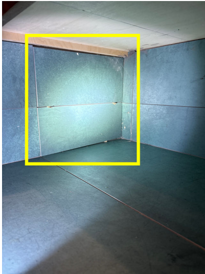
Missing grout -half bath
