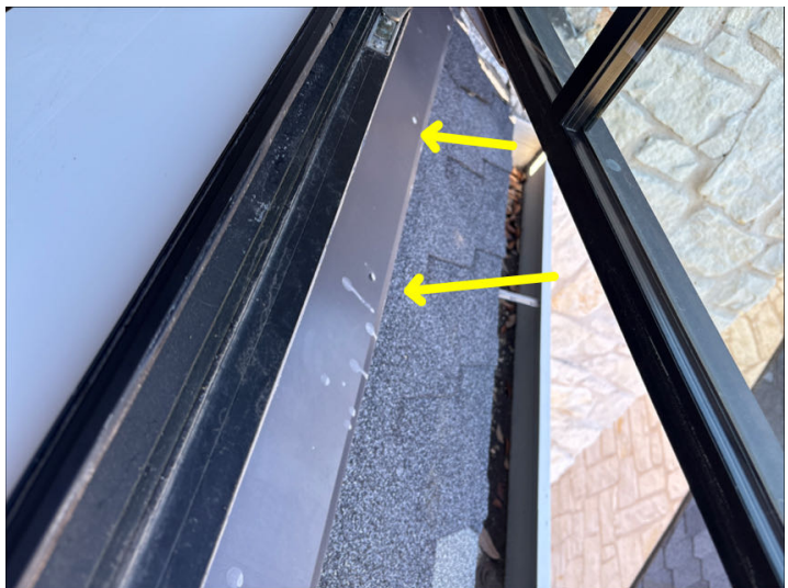
UNSEALED FASTENERS -third floor below windows
