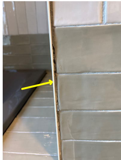
GAPS / CRACKS AT SHOWER
