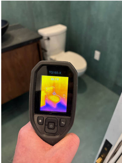
NORMAL THERMAL READINGS - DRAINS
