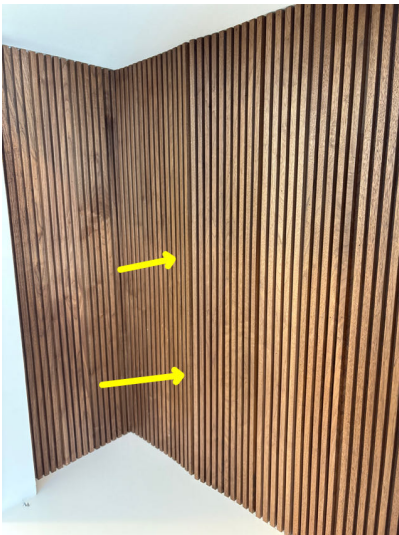
Accent wall is loose
