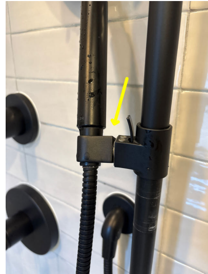
Damaged wand holder
