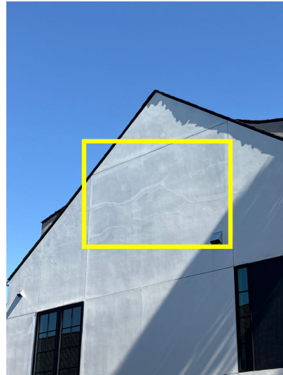
Large stucco cracks
