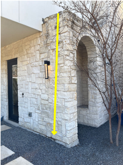
Water penetrating through horizontal masonry and coming out of weep holes
