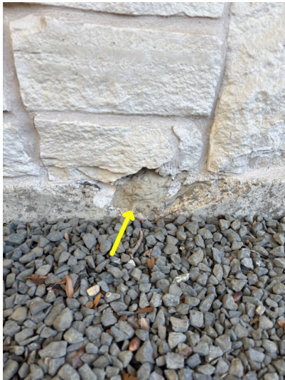
Previous repair near front door -consult owner as needed
