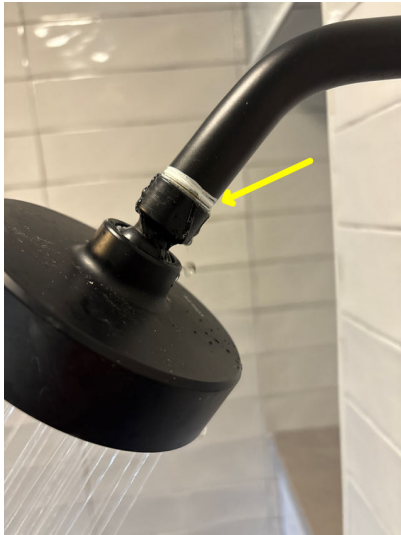
Shower head leak
