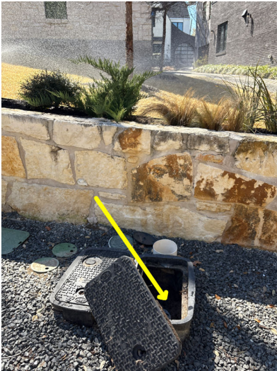
Meter and shut off for unit 1
